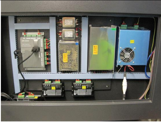
Power supplies and controls
